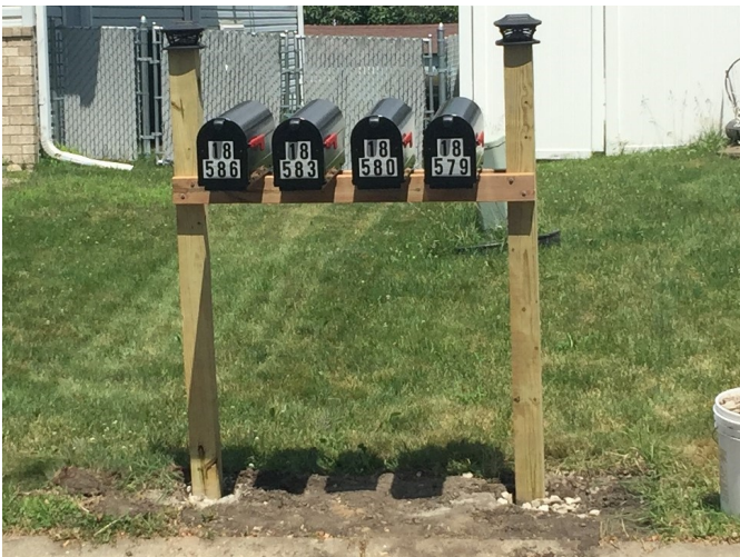
Son Christopher tore out old boxes and dug the holes for the concrete footings. New boxes and solar lights on top. Neighbors and mail lady love me.
